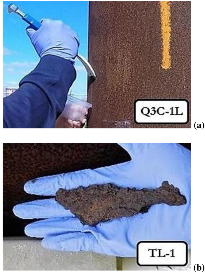
Figure 6.4 Collection of surface oxide samples: (a) scraping of patina to obtain powder sample; and (b) pack-out rust sample removed by hand from junction box area of Pole TL-1.
