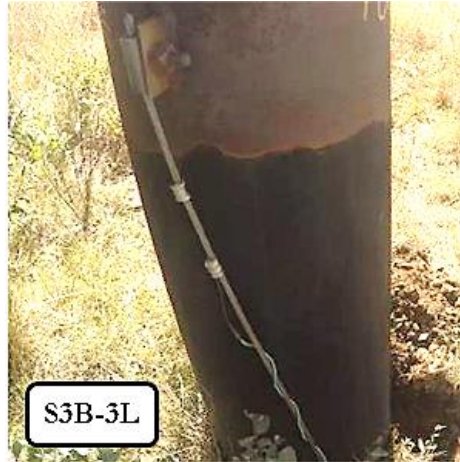
Figure 3.16 Pole S3B-3L showing minor coating delamination but overall dense and adherent patina.
