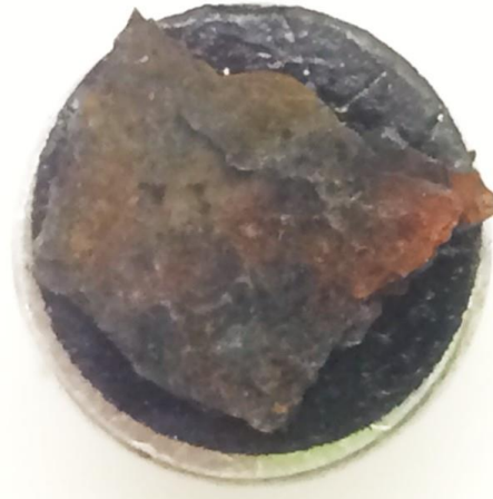
Figure A.11 Loose rust sample from GS fastener region of Pole 8Z-2L at Site 5.
