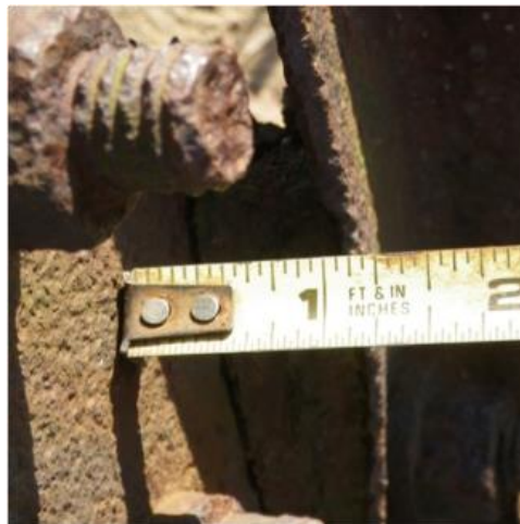
Figure 2.8 Pack-out damage at connection in WS transmission line lattice structure. Note bent steel member.
