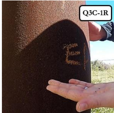
Figure 3.11 Non-adherent patina sloughing off with light rubbing of pole wall surface.
