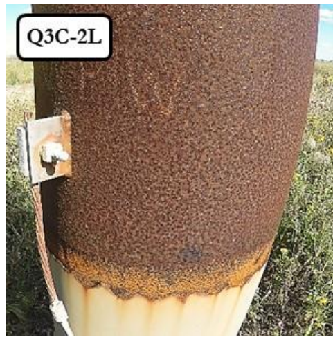
Figure 3.8 Corrosion prevention measures seen on Site 2 poles, including GEC link to grounding rod and magnesium anode connection.
