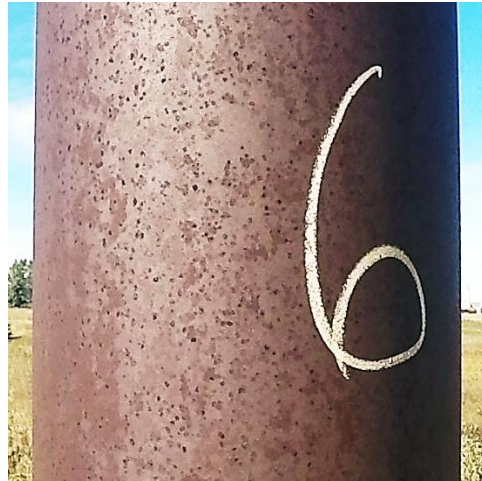
Figure 2.9 Widespread pitting over surface of WS pole wall.
