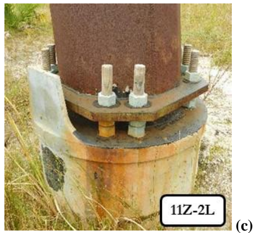
Figure 3.29 Visual assessment of poles at Site 5: (a) discolored patina, corroding fasteners, and vegetation build-up around Pole 8Z-2R; (b) uniform patina but corroding fasteners on Pole 11Z-6R; and (c) uniform patina and GS fasteners on Pole 11Z-2L.
